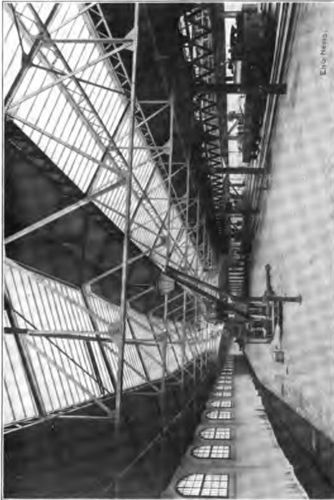
Fig. 155. Interior View of a Freight Shed Showing Steel Roof Trusses with Wide Spacing and Riveted Truss Purlins.
